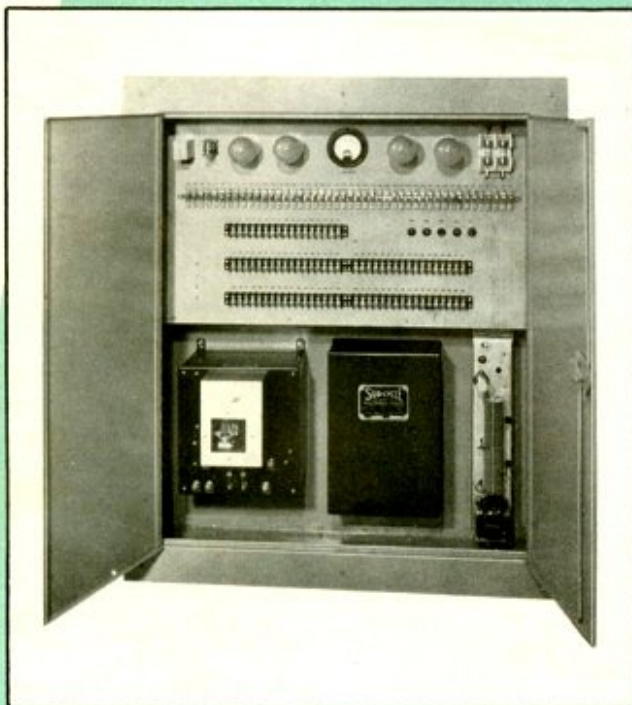
Power distribution board
